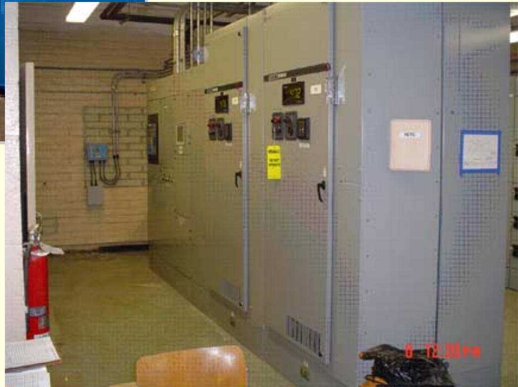
Fig. 5.14 Electricity distribution and control room (MDB + PLC)
