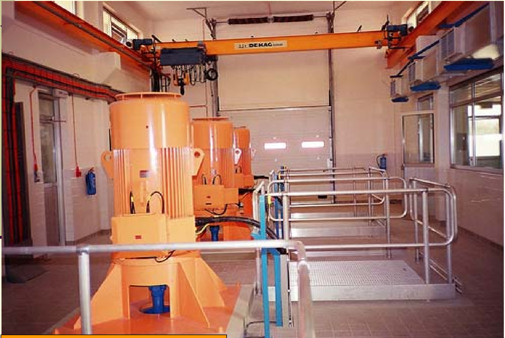
Fig. 5.10 Dry room for dry pumps
