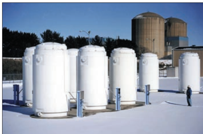
TN-40 Dry Storage Cask
