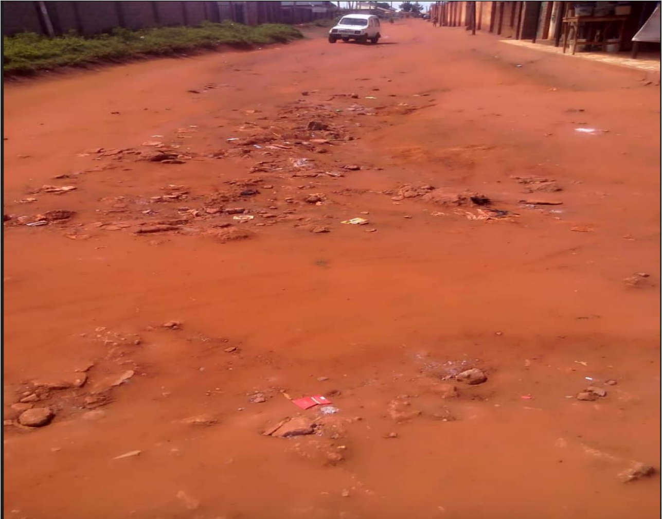
Figures 6 & 7: Parts of Afaka community access road
