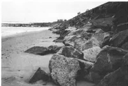
Figure 6. Displaced stones after severe storms.
