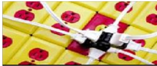
Overloads are a major cause of fires.
