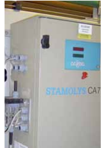
Precise control of silica to protect the turbine
