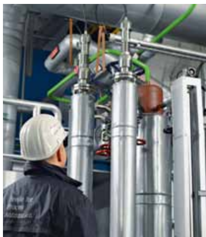
Guided Wave Radar (GWR) level measurement (sensor remote) at low pressure preheater. Safety shutdown system 2 out of 3 voting architecture (2oo3 redundancy)
