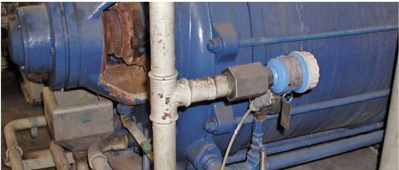
Liquiphant installed to protect the pump from running dry
