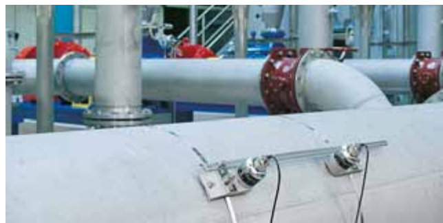
Prosonic Flow (clamp on version shown) is used to control cooling water for the condenser
