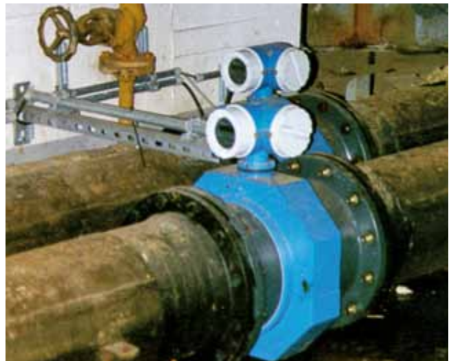
Promag electromagnetic flowmeter registers the cooling water volumes
