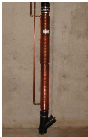
Figure 25: Installation of a Double-walled Copper-on-copper Heat Exchanger in a Vertical Section of the Master Drain Line in a Canadian Home (2007) (Source: Wikimedia Common) 31
