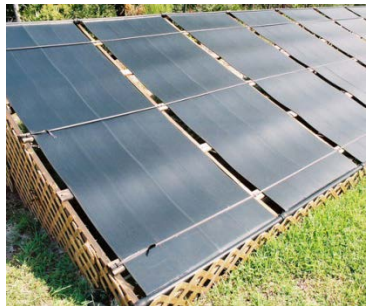
Unglazed liquid collectors 45
