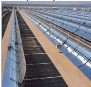
Parabolic solar concentrators 46
