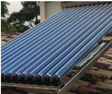
Evacuated tube collectors 42
