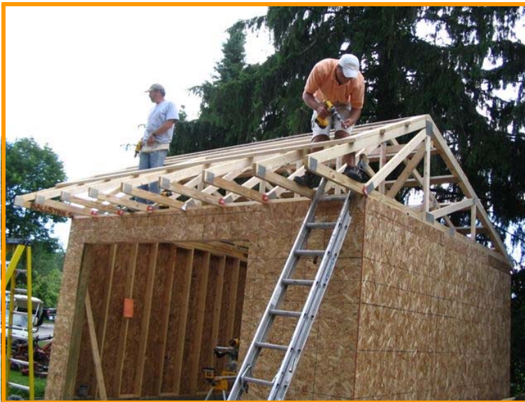
Randy Alexander, Bill Martin and Steve Ludwin donated their time and skills in the construction of the pesticide building.
