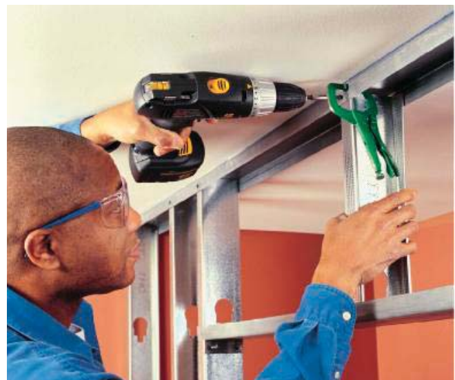
(Fig. 14) After setting the guide tracks the studs are attached to create the walls.
