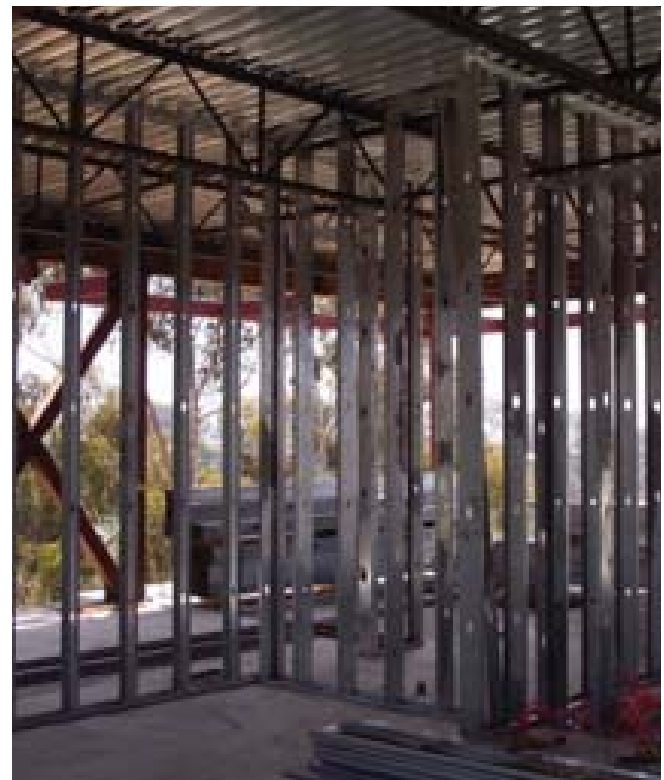
(Fig. 16) A steel-framed wall system tied into steel floor trusses and steel pan flooring.
