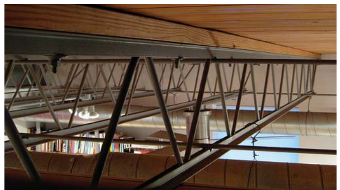
(FIG.C) TRUSSES offer a speedy alternative to traditional lumber joists in both floor and roof systems bridging larger spans and flexibility in the running of MEPs.
