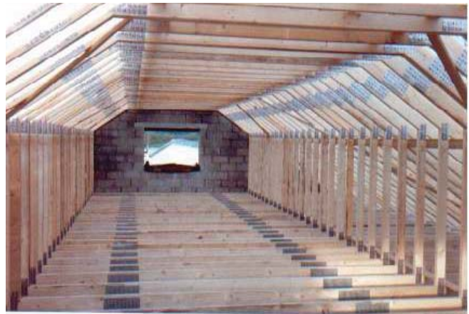
(Fig. 27) Roof trusses can be configured in many different ways to account for ventilation, storage, or mechanical systems.
