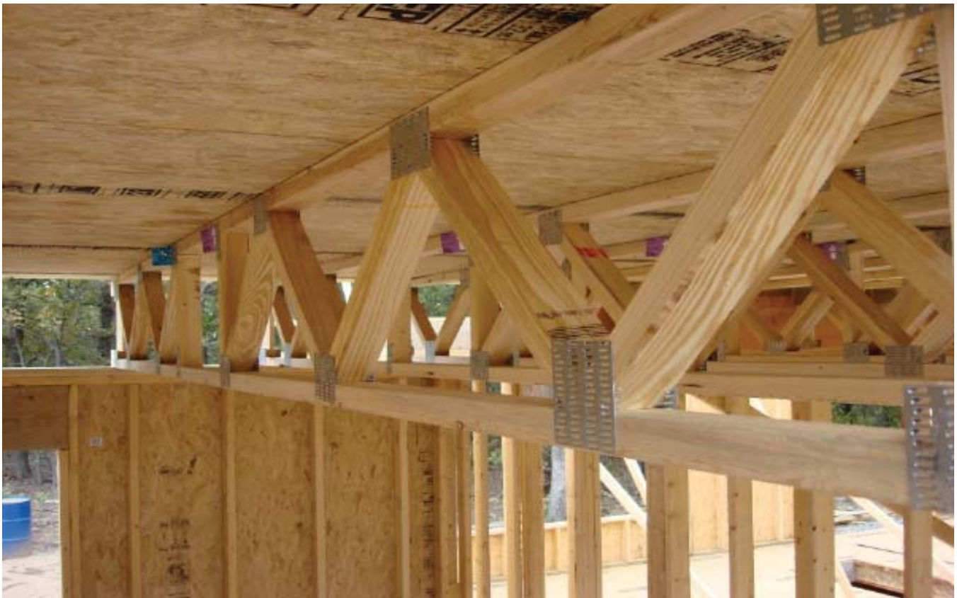
(Fig. 20) A truss used to create a platform-framed second floor. Gaps in the truss allow room for plumbing, electrical, and HVAC to run freely.
