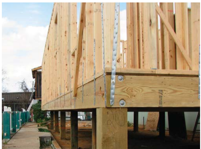
(Fig. 4) It is important to ensure studs are properly strapped according to local building codes to prevent failure in a high wind event.
