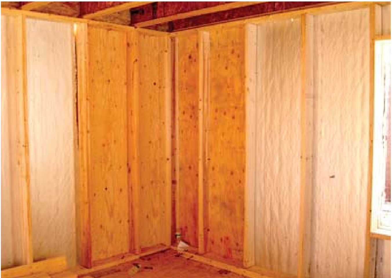
(Fig. 8) 2x6 studs on 24 inch centers, stack framed, single top plates, two stud corners, no jacks, no cripples. Almost 40 percent of the framing elements typical in traditional wood frame construction have been removed.
