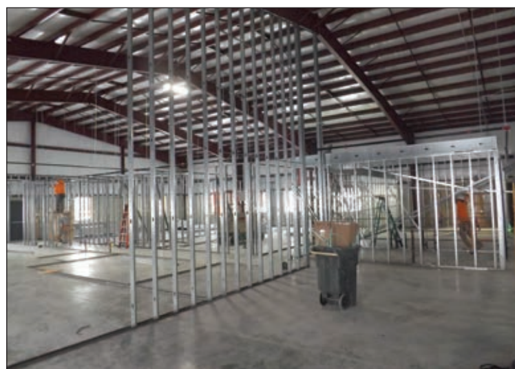
Workers construct framing for classrooms, community rooms, and office space in the new community center at the Clark.
