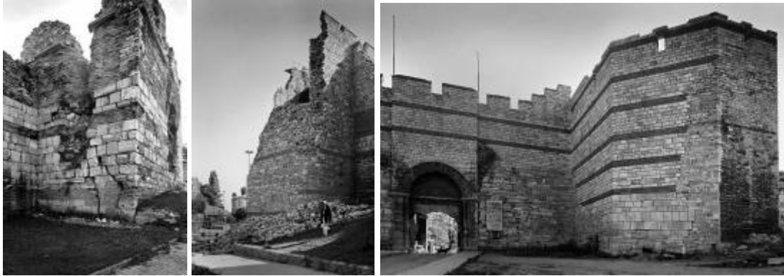
Figure 5: (a) Original section of Theodosian City Wall, Istanbul after 1999 earthquake. (b) Modern reconstruction of a part of the City wall that collapsed during 1999 earthquake. (c) Modern “restoration” work shows the artificial look that results when the work is conceived without its original structural rationale.
