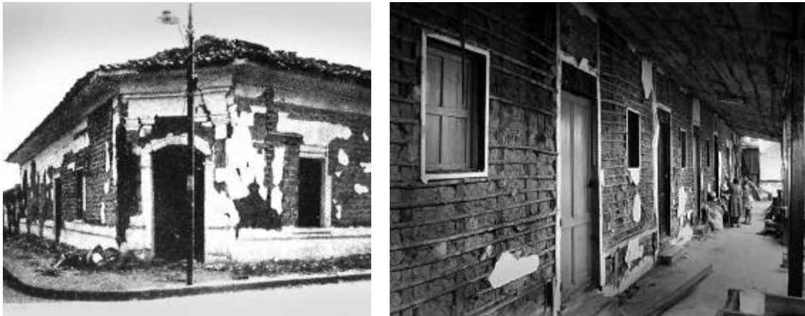
Figure 11: (a) J.R. Freeman's photo of Taquezal building in Managua after 1931 earthquake. (b) San Salvador Bahareque building after 1986 earthquake showing a similar plaster shedding.
