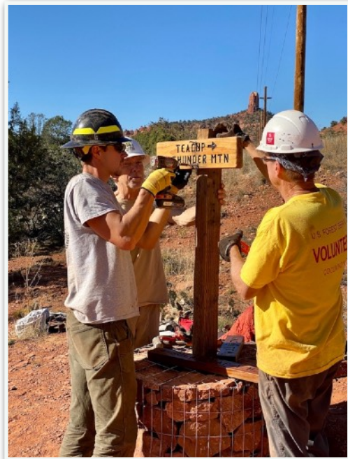
New rock cairn and sign installation by Matt (USFS), Rich Spinelli and Rod Cashin
