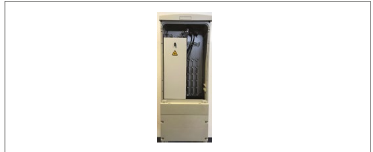
GF-NVT in KVZ92
