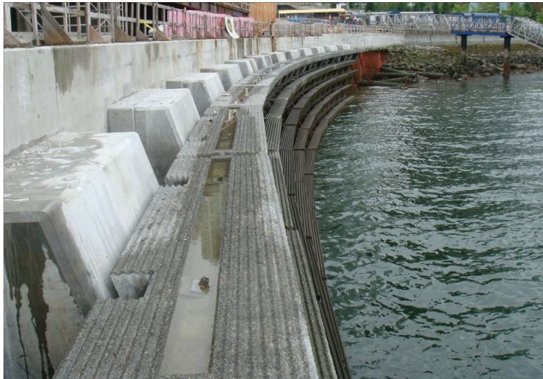
Figure 3. Habitat skirt constructed through a joint effort by DFO, Tetra Tech EBA and WorleyParsons Westmar along the shores of the Vancouver Convention Centre (Image Source: https://blogs.ubc.ca/vcchabitatskirt )
