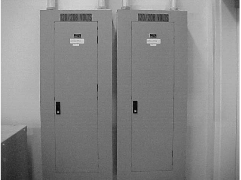
Figure 8-6. Electrical panel on right trips prematurely.
