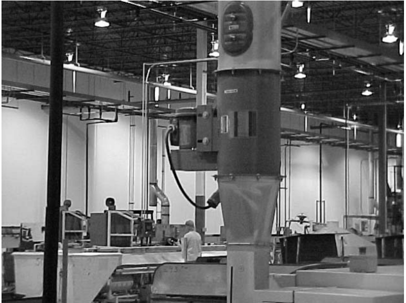
Figure 8-2. What would cause this 1 HP fan to have a high failure rate?
