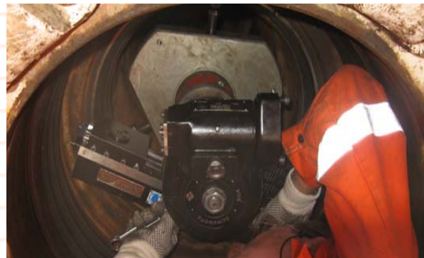
Machining inside wellhead
