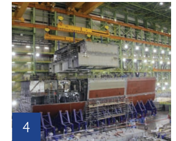
4 Progress continues at Halifax Shipyard with another level added to the mega-block
