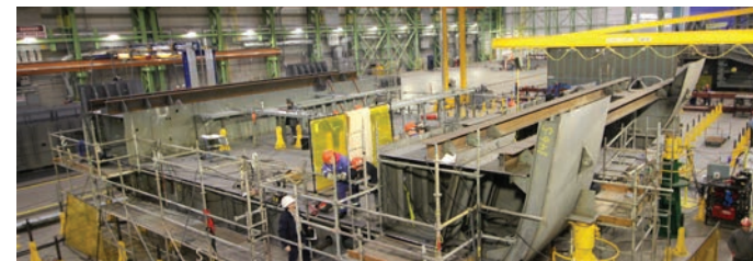
Approximately 300 kms of cable will be installed on the first AOPS vessel, equivalent to the driving distance from Halifax to Yarmouth, Nova Scotia
