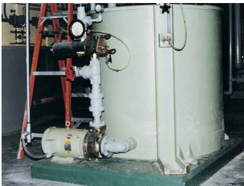
Reverse osmosis, Ósmosis invertida
