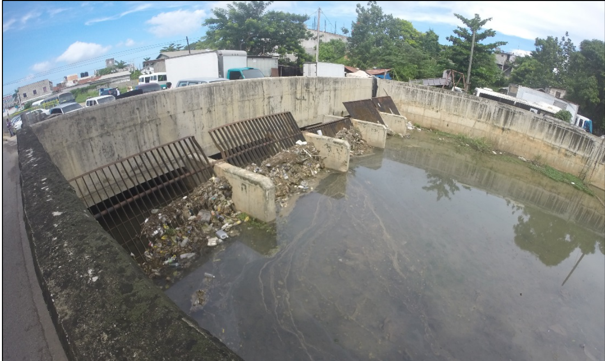
Figure 13: Garbage in the South Gully, Montego Bay
