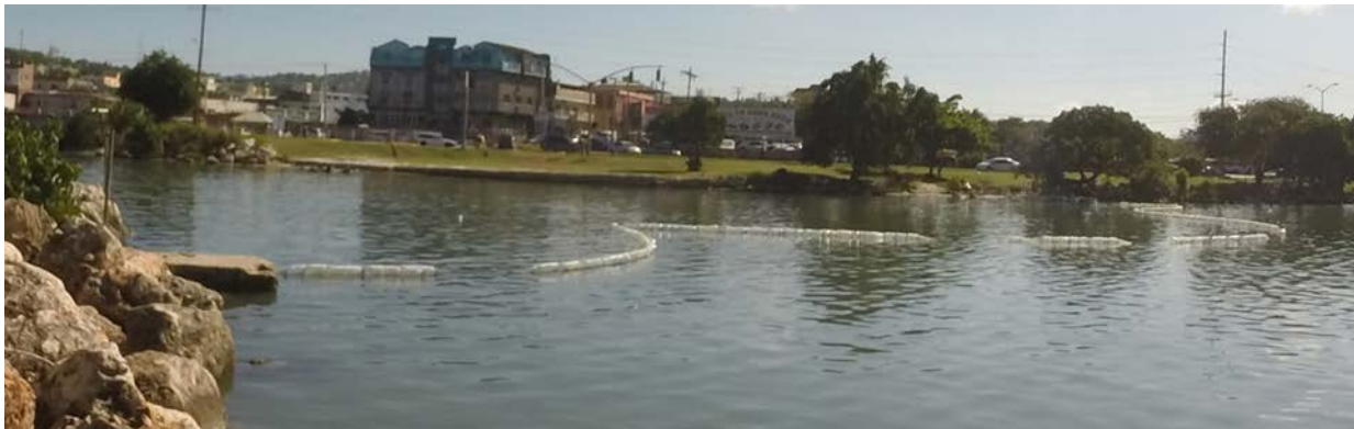
The boom in early January 2016 illustrating minor damage - one section of the boom was loose
