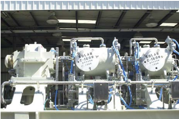
Figure 23. Centrifugal Compressors for Re-Injection Duty at 240 bar (3,500 psi) Discharge Pressure
