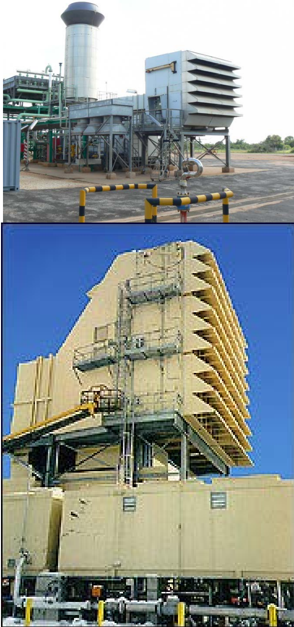
Figure 7. Gas Turbine Filter House
