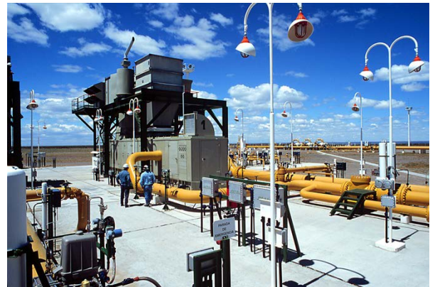
Figure 5. Fully Enclosed Gas Turbine Installation
