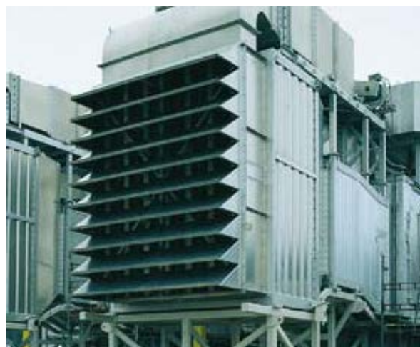
Figure 11. Weather Hood on inlet Filtration System
