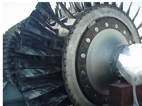
Figure 3. Oily Deposits on Axial Compressor Blades from No. 1 Bearing Oil Leakage on a Large Heavy Duty Gas Turbine.
