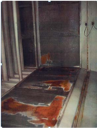
Figure 35. Corroded Floor of Inlet Duct (Clever, 1988).
