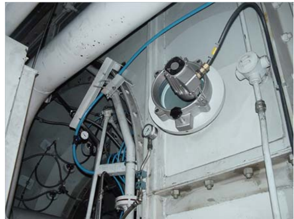
Figure 47. Illuminated Viewing Window on a 123 MW Gas Turbine.
