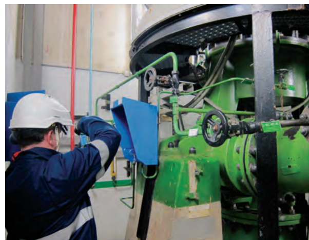
FIG. 1. An Agency reviewer in an OSART follow-up mission assessing the functionality of an essential service water pump at the Gravelines nuclear power plant in France.
