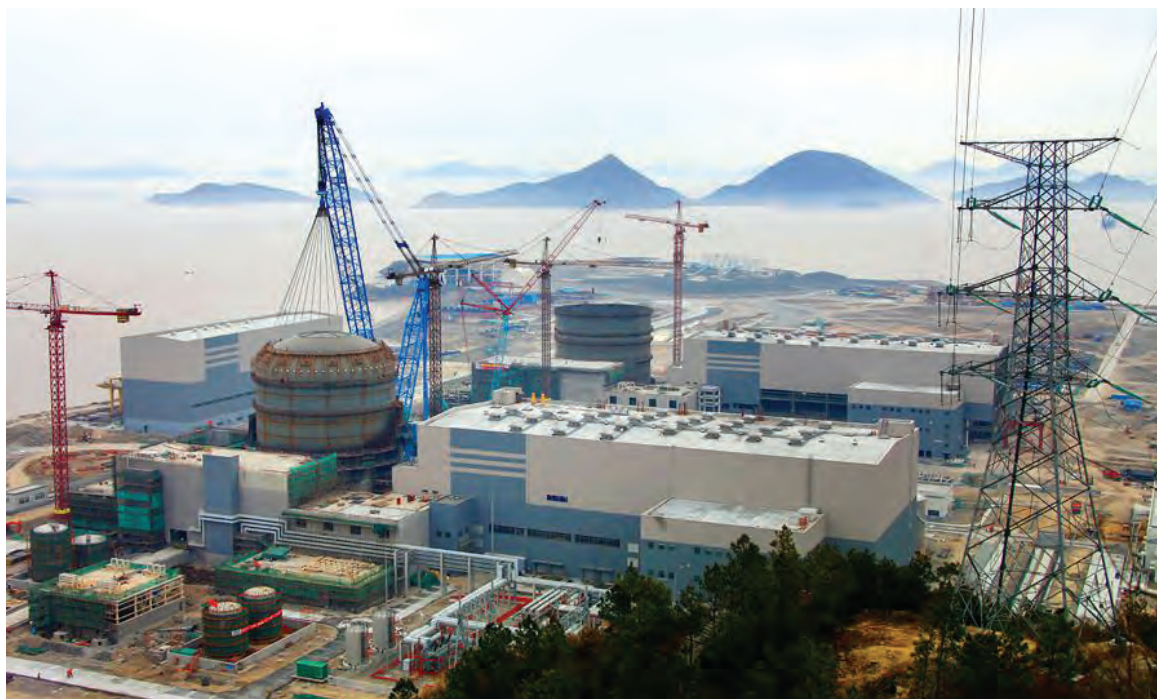
FIG. 3. Installation of the containment cap for a unit at the Sanmen nuclear power plant, one of the many nuclear power plants under construction in China, a country with an expanding nuclear power programme. (Photograph courtesy of CNNC.)
