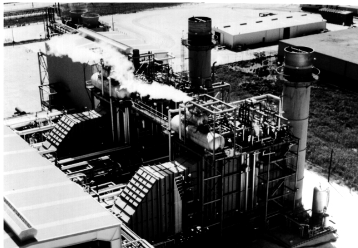
Figure 23. Two natural-circulation HRSGs operating with MS7001EA gas turbines
