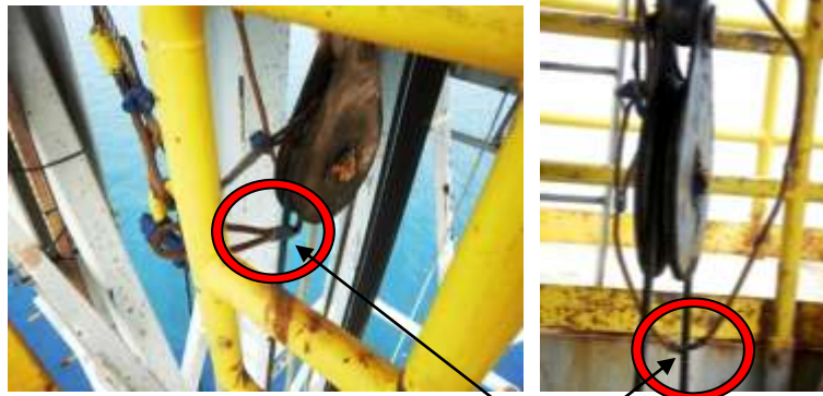
Safety slings attached to the sheaves are seen rubbing against the slings passing through the sheaves. These should be diverted to avoid damage to either sling.
