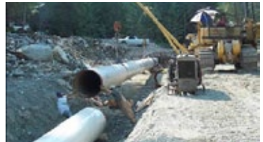
Figure 12. A Penstock Pipe for a 5-10 MW hydropower project. Courtesy of Cloudworks Energy Inc.
