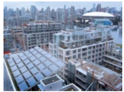
Figure 14. Roof-mounted solar PV panel.
