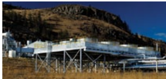
Figure 9. Electricity is generated from recovered heat at this natural gas compressor station in Savona, B.C.
