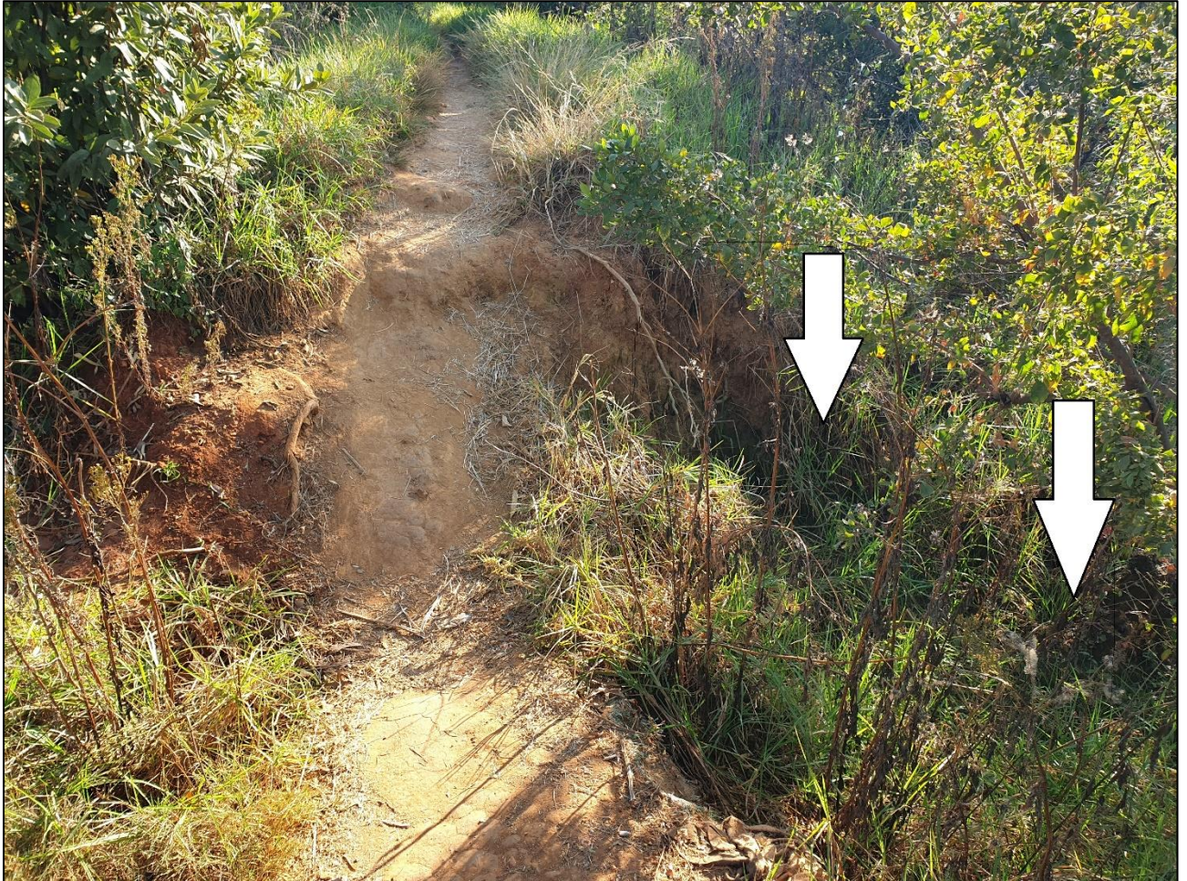
Figure 3: Close up view of the breach section – in the vicinity of AFD TP7. Arrows indicating approximately where water flow was noted – although clear view is obstructed by vegetation
