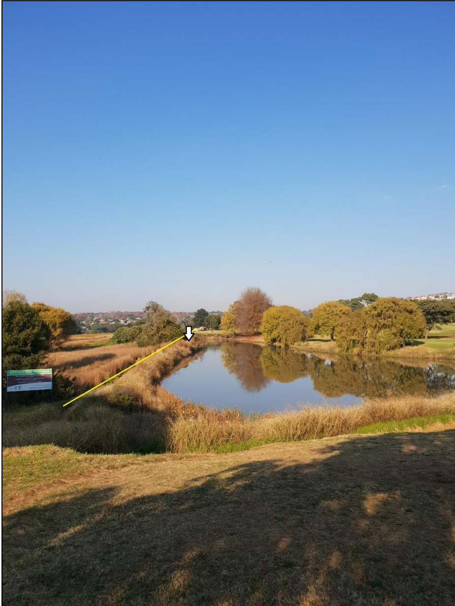
Figure 2: View of the dam from the north (approximate centre line and position of breach are shown by yellow line and arrow, respectively)
