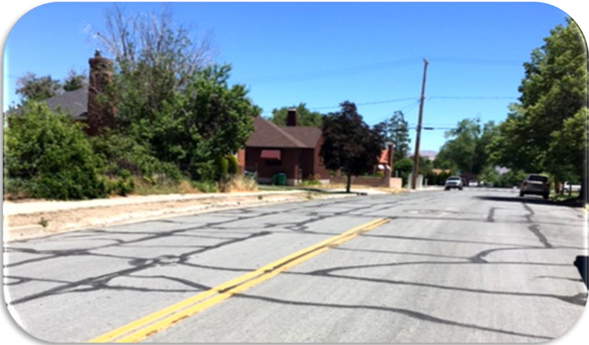
Photo #1 - Taylor Street east of Gordon Avenue. Note block cracking
