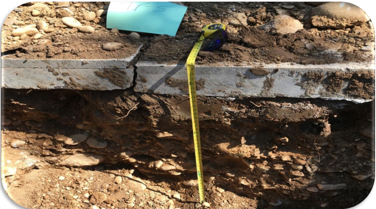
Photo #4: Trench sidewall at Test Pit TP-5 (Reno Avenue). Note pavement overlying concrete and displacement at the joint. Structural section directly on underlying clay soils.
