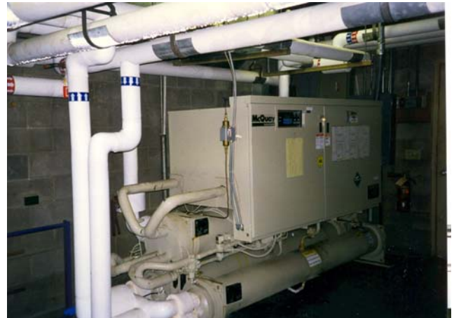
Figure 3. Photograph of one of the water-to-water heat pumps at the Inn of the Seventh Mountain.
