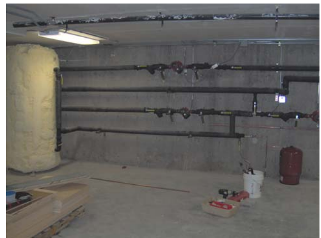
Figure 4. Photograph of the mechanical room, showing the distribution piping and storage tank.
