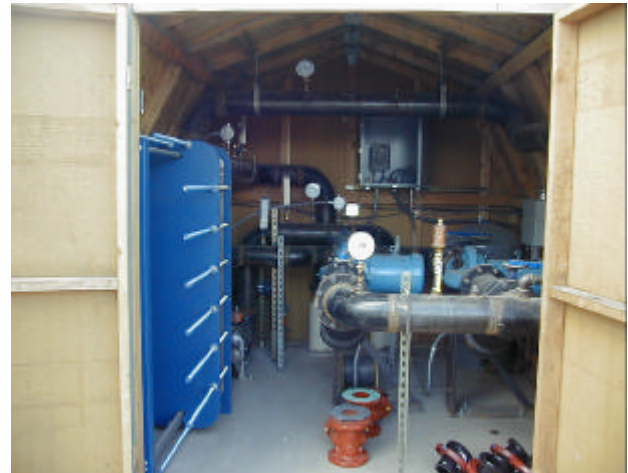
Figure 3. The main plate heat exchanger.
