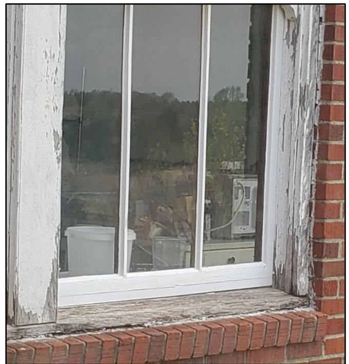
Damaged window frame to be restored
