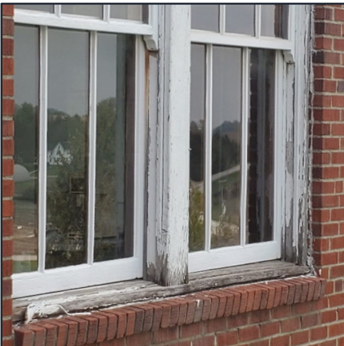
Damaged window frame to be restored
