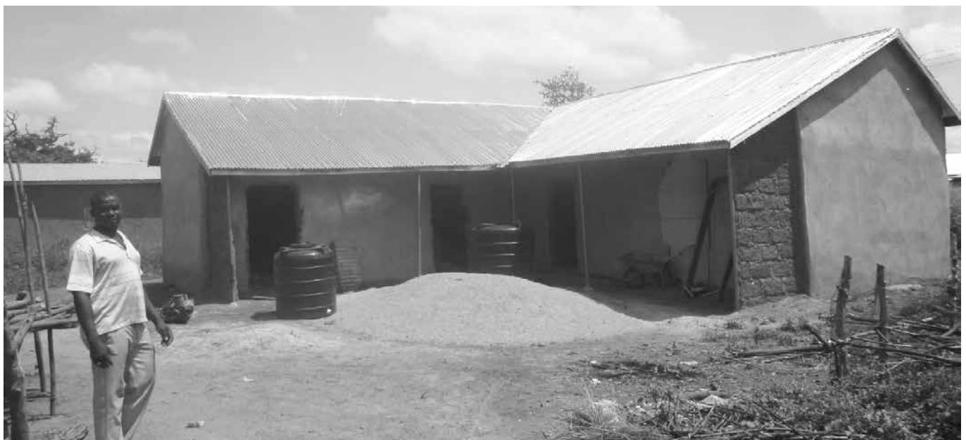
Above right: Alhassan Salifu Baako (GSA Rep), Adam Hizikil (HT) and Yakubu Abukari (PTA Chair) at partially built teachers’ block at Tibung JHS. Above: The almost completed teachers’ accommodation
