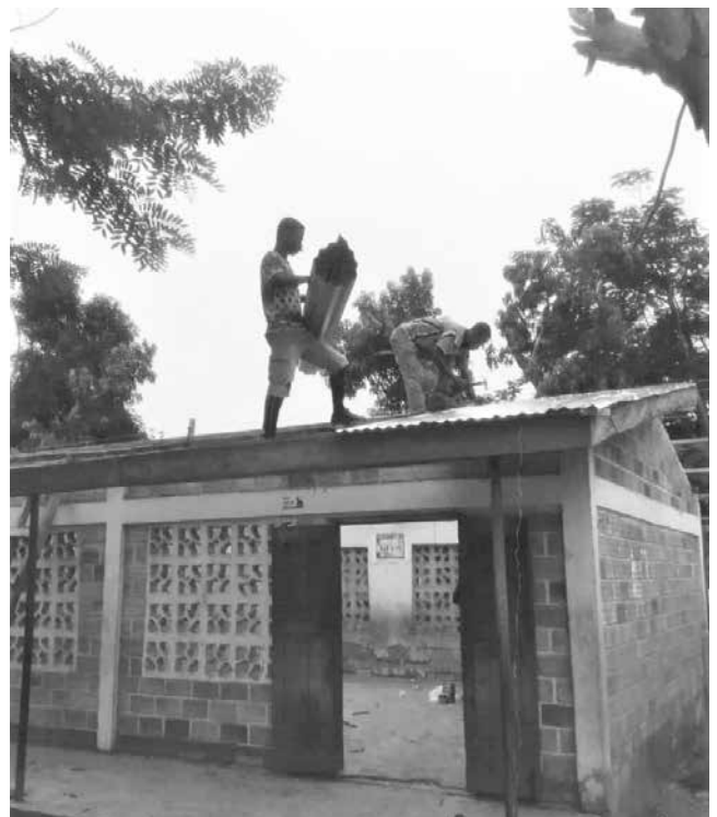
Top: Kenyasi No 1 Basic School showing the old rusty roof. Above: The new roof being repaired
