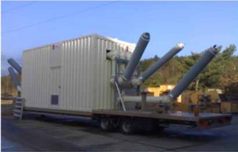
Algeria – 245 kV mobile substation
