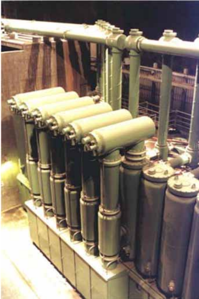
Canada - 330 kV - 140 m below the ground surface
