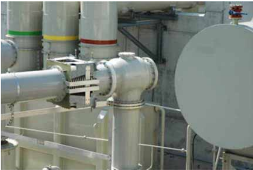
Direct transformer connection with adjustment bellow
