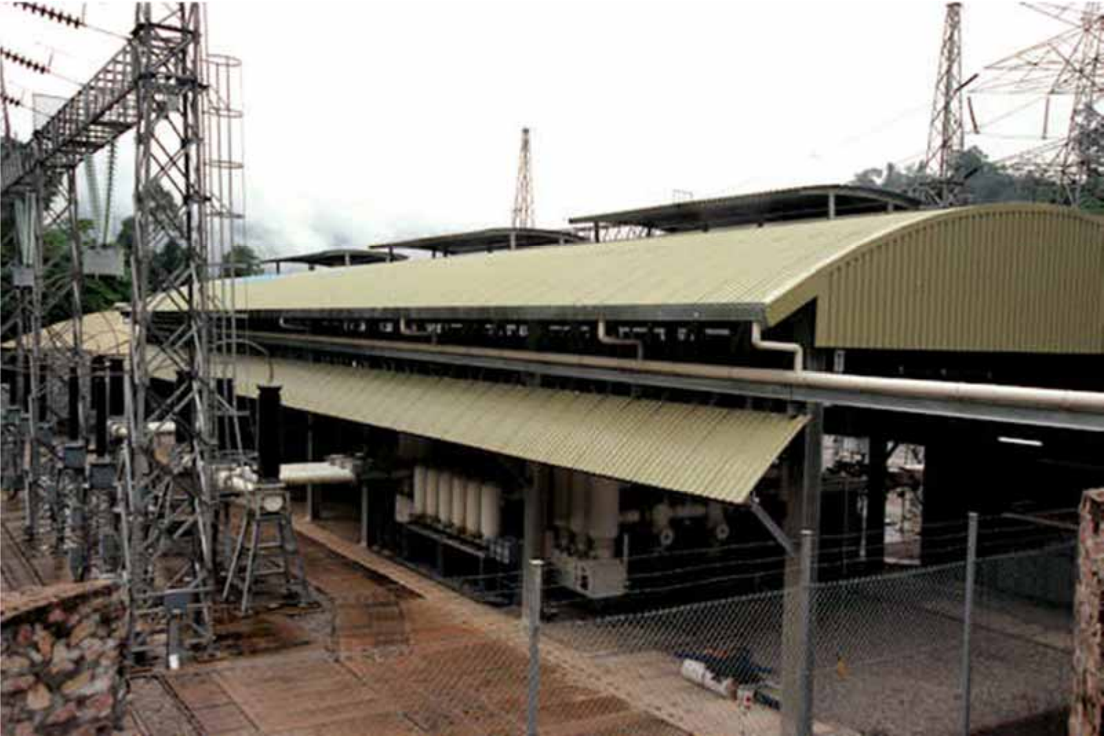
Malaysia – Pergau – 245 kV
