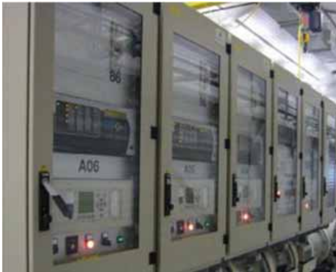
Canada – Jackpine – Protection relays in integrated LCCs
