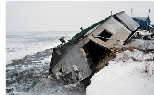
An abandoned house at the west end of Shishmaref, Alaska, that slid during a storm in 2005. Residents have voted in favor of relocating the community to the mainland. Credit: Diana Haecker/Associated Press
