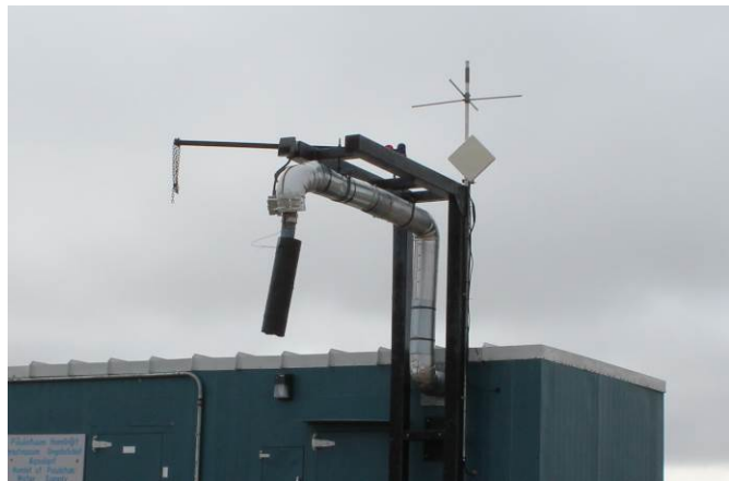
Figure 10.1 – Overhead Fill Arm
