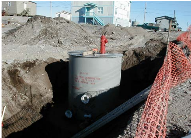
Figure 5.5 - Hydrant Access Vault
