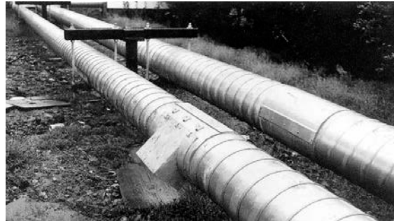
Figure 3.2 - Typical Aboveground Pipes in Inuvik
