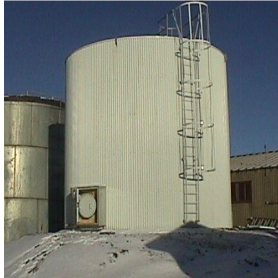
Figure 16.1 – Aklavik Water Tank
