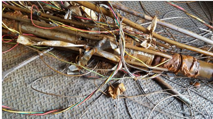
Figure 7.4 - Intake Pump With Tape
