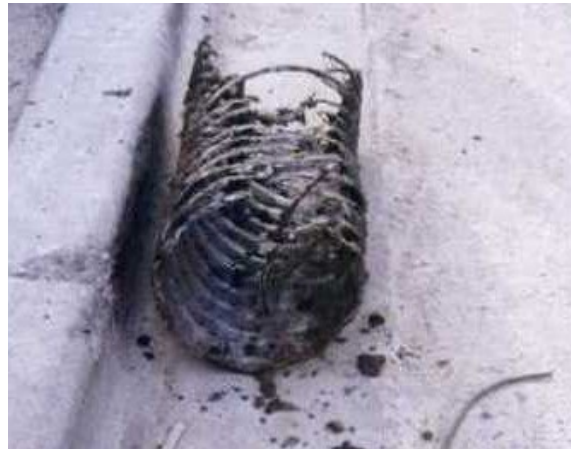
Figure 3.1 - Corroded Corrugated Metal Pipe
