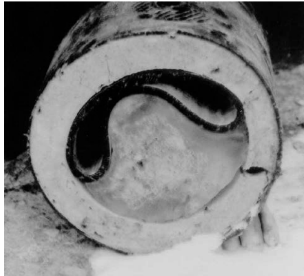
Figure 3.3 - Collapsed HDPE Pipe
