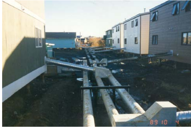
Figure 3.8 - Aboveground Piping in Inuvik Using Individually-Insulated Pipes
