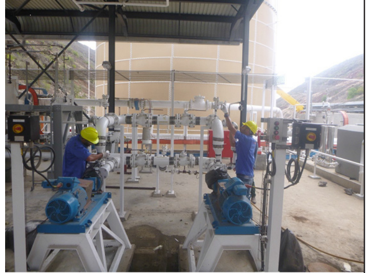
SmartJet performing air leak test on aviation fuel pipework at the Bulk Fuel Installation loading bay, March 2019
