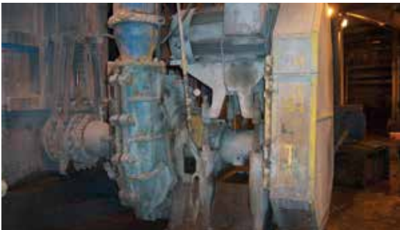
SRL-XT 14×12–36 on Ball Mill Discharge Service
