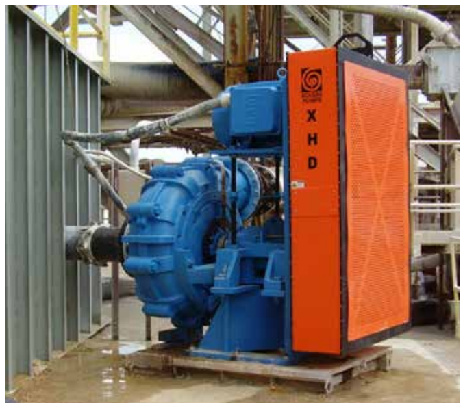
Primary Sand Slurry Pump in an Aggregate Plant
