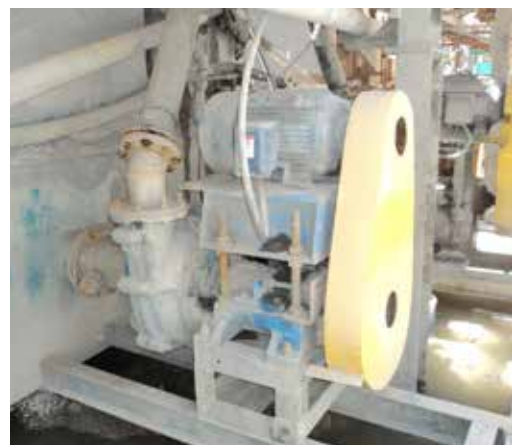
Mill discharge in silver plant
