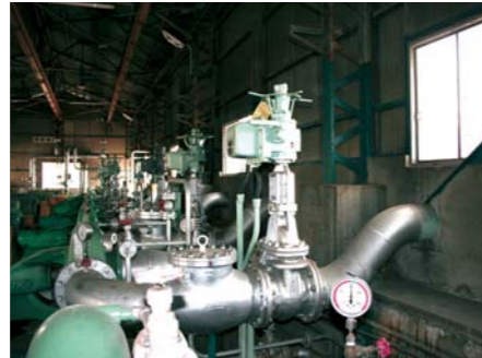
Cooling water supply unit
