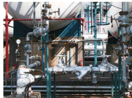
Drain transfer unit
