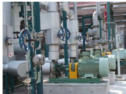
Plant cold water unit
