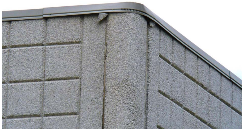
corner panel failures of various degrees
