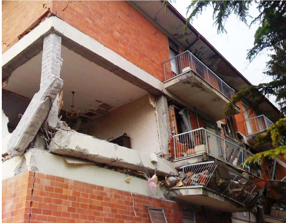
squeezed-in soft storey
