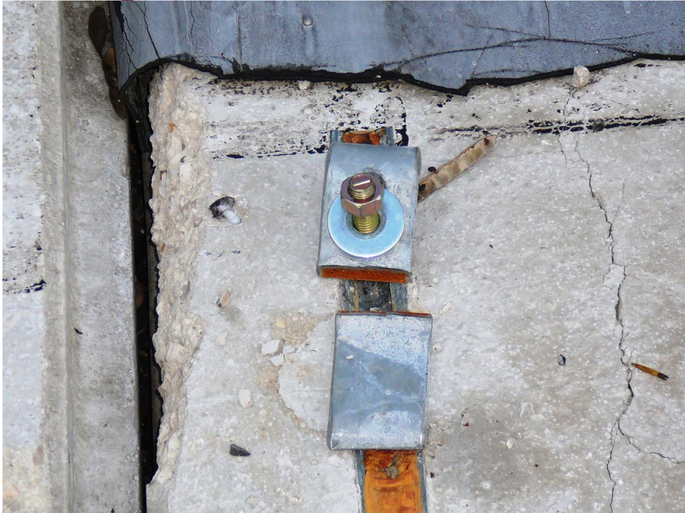
Fastener plate of wall panel failed by unforeseen action
