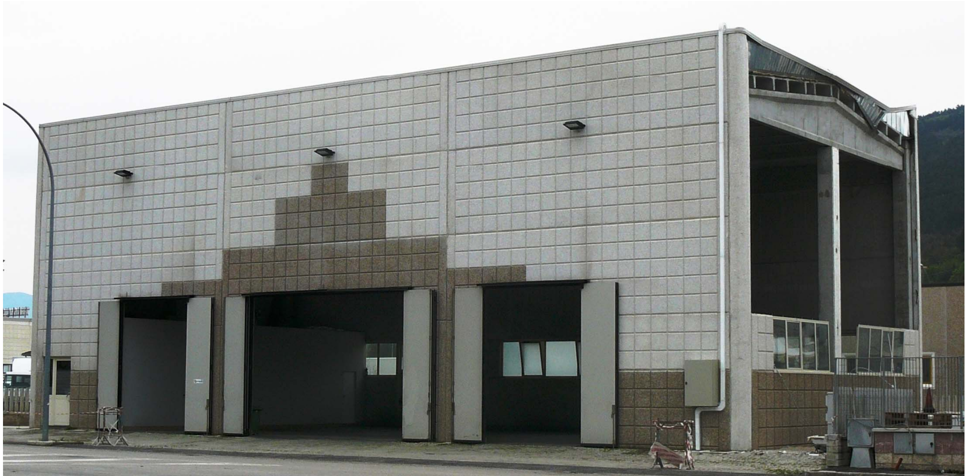
fallen façade of horizontal panels (right-hand side)
