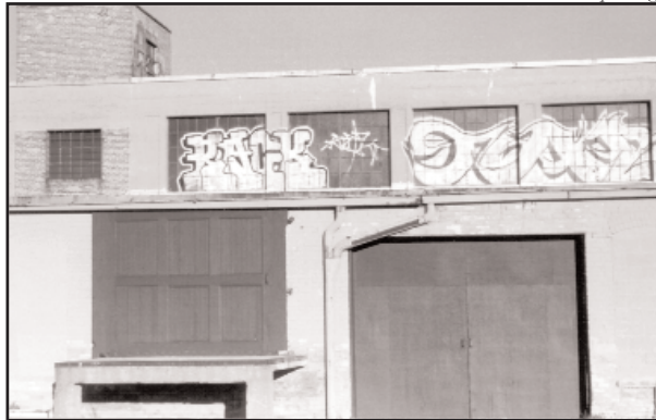
Graffiti often appears in hard-to-reach yet highly visible locations, such as on the upper-story windows of this warehouse.
