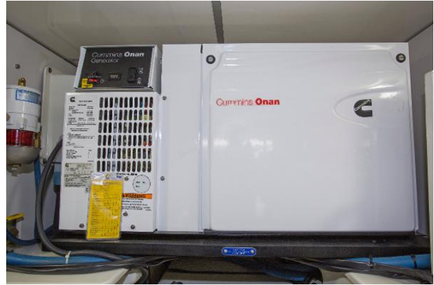
Quiet ONAN Generator In Soundshield
