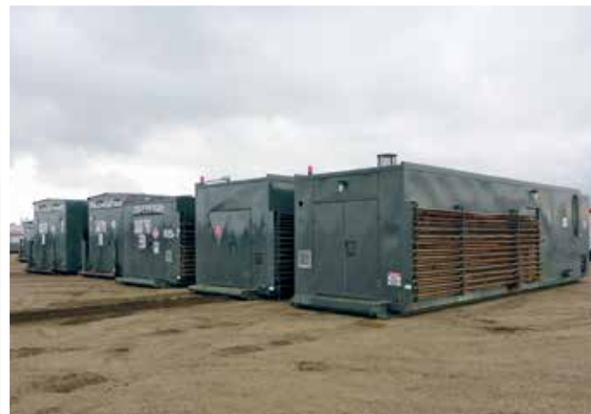
5 of 7 - Saskatoon, Smith & Williams & Davis Boilers
