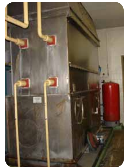
One of the Air Conditioning Cooling Towers
