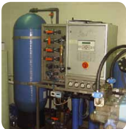
Inside the Desalination Plant
