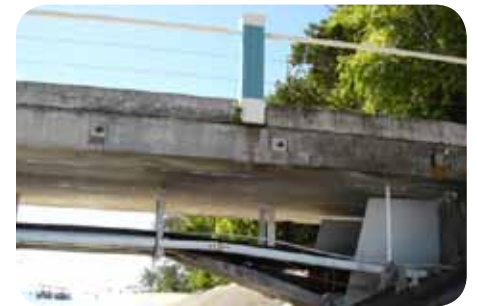
The water pipe runs under the jetty to the resort.
