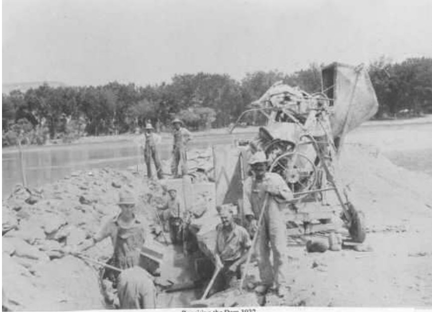
Repairing the Dam 1932 Supervised by George Thurman Left front facing camera, Hawley Seely, at Hawley's right, John Vetere Sr., 3 rd on right, Clifford Phillips; 4 th on right, Joe Chido. Remainder unidentified.
