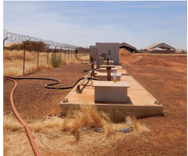
Photo 4. Water treatment infrastructure streaming to a water pool at Camp Castor, Gao, Mali, 2016. Malkit Shoshan/FAST.
