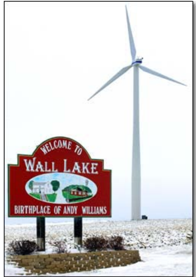
660 kW Wind Turbine Owned by Wall Lake, Iowa 6
