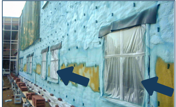
Typical masking off of windows prior to the installation of spray polyurethane foam.
