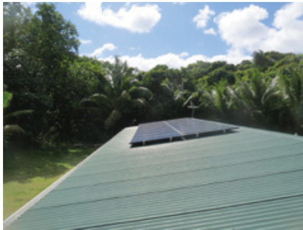
Figure 6: Array on House Roof
