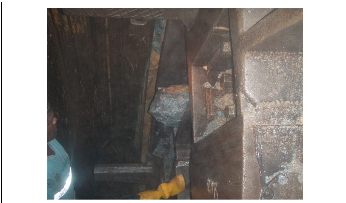
Figure 8.3 Example of Rock Fragment Trapped in the Opening of the Cutterhead
