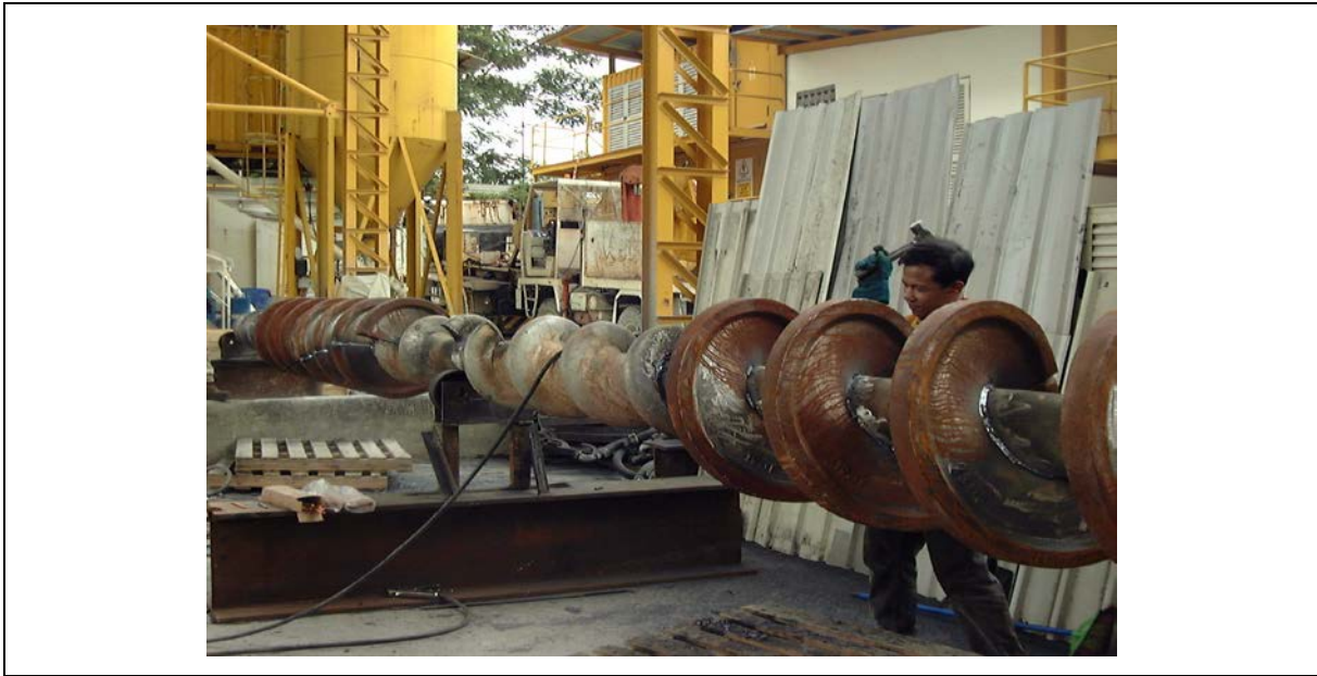
Figure 4.6 Example of Excessive Wear on Screw Conveyor
