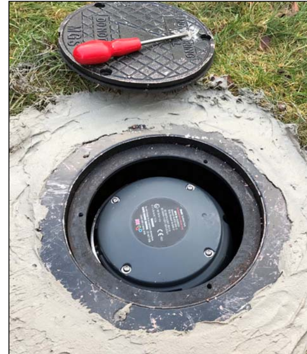
2 nd Generation On-borehole device Gas Sentinel ®
