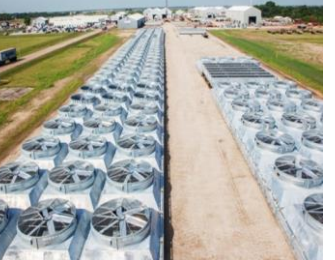
Air Cooled Heat Exchangers
