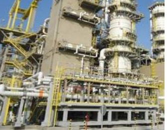
Gas Pre-Treatment and Nitrogen Rejection Units
